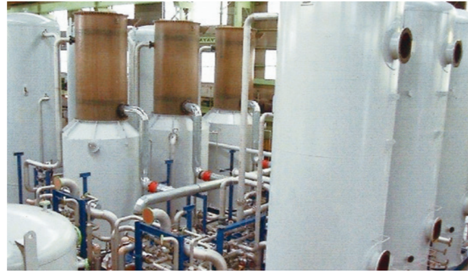
DEMINE SKID [2,500 φ ×5,900 H 3基 2,500 φ ×3,970 H 3基 2,500 φ ×6,200 H 3基]
